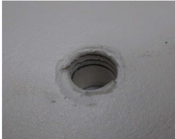
Picture - 2 - Cracks (Ø9,0 test)
